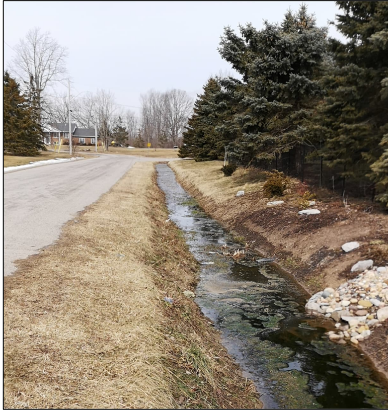
Figure 6 Bell Acres Roadside Swale
