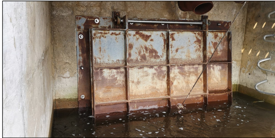
Figure 5 OMC Outlet Flap Gate
