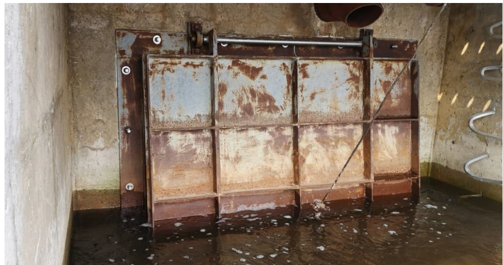
Figure 25 Oil Mill Creek Flap Gate
