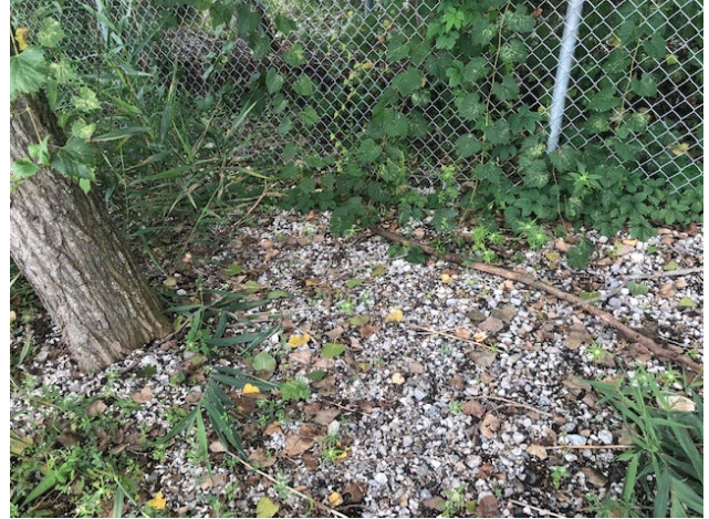
Photo 13: Gaps at the base of the fence
