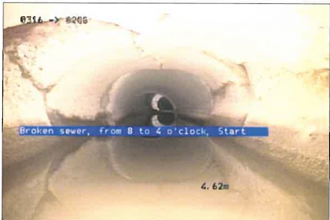
Figure 2-7 Partially Collapsed Sewer on Omer Avenue
